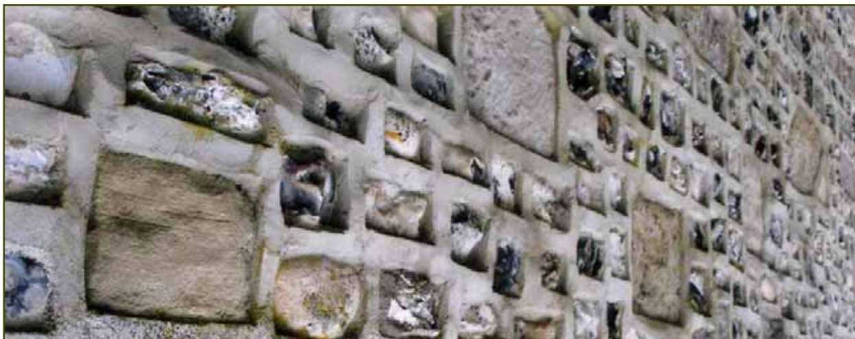
Figure 23. An example of poor repairs to a stone wall. This form of 'strap pointing' is aesthetically unattractive, is not a tradition of the area and will accelerate the degradation of the wall
